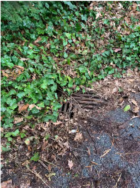
Catch Basin at South Side of SE 32 nd Street, At Point K
