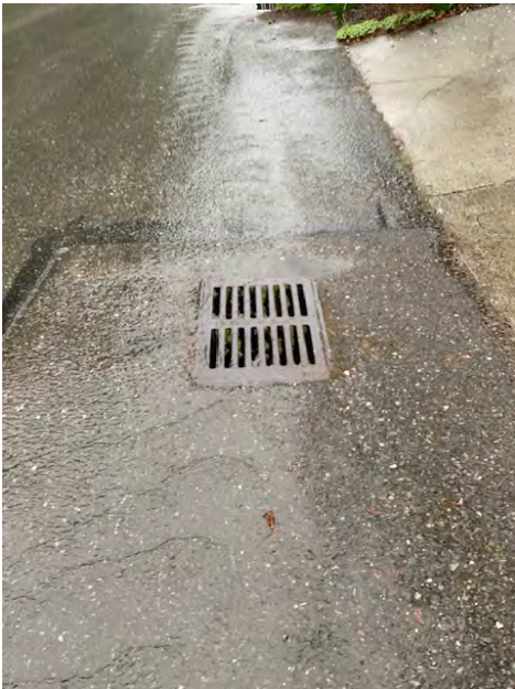
Catch Basin along Noth side of SE 32 nd Street, Downstream of Point H
