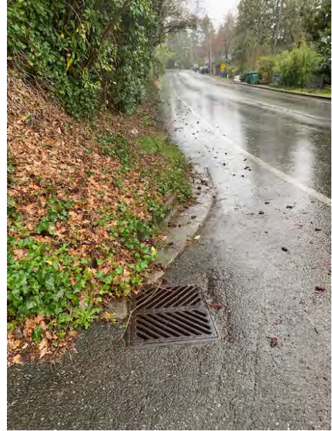
Catch Basin At East side of W Mercer Way, At Point L. End of Analysis Looking Downstream
